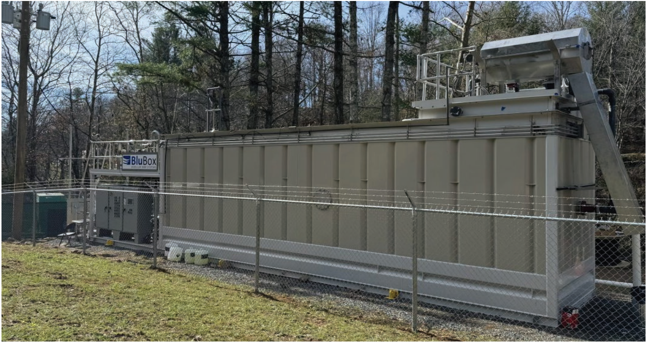
FIGURE 9. BluBox Mobile Wastewater Unit in Town of Spruce Pine
