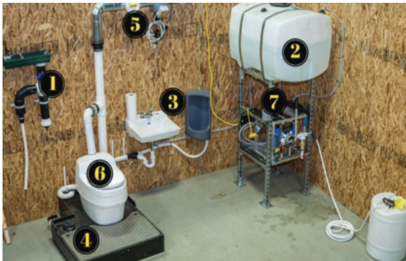
FIGURE 10. Portable Alternative Sanitation System
