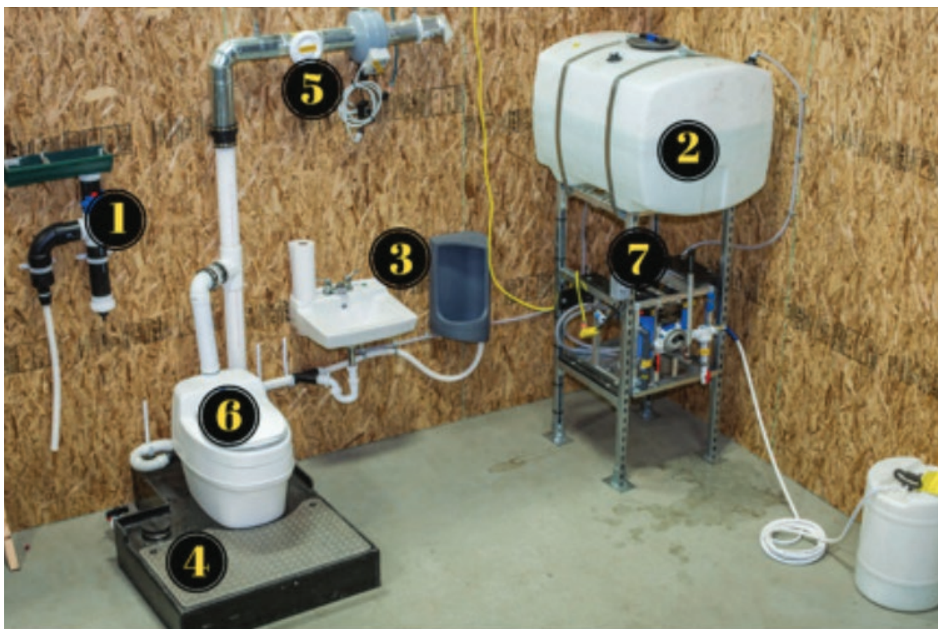
FIGURE 7. Portable Alternative Sanitation System
