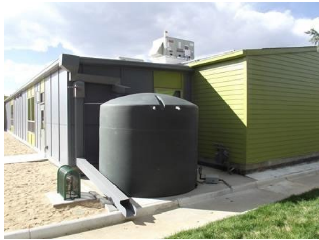
Photo 4. Cistern at Denver Green School. Source: Holly Piza
