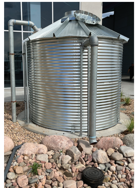
ES Photo 1. Cistern at the CSU Spur Campus. Source: Jane Clary
