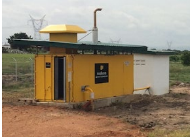
Generator container and grid switchboard
