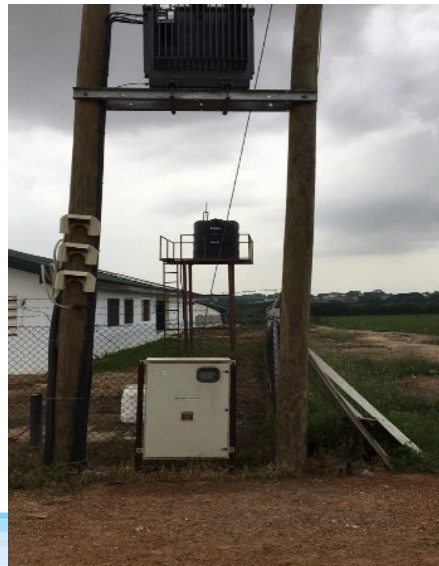
Meter and grid connection
