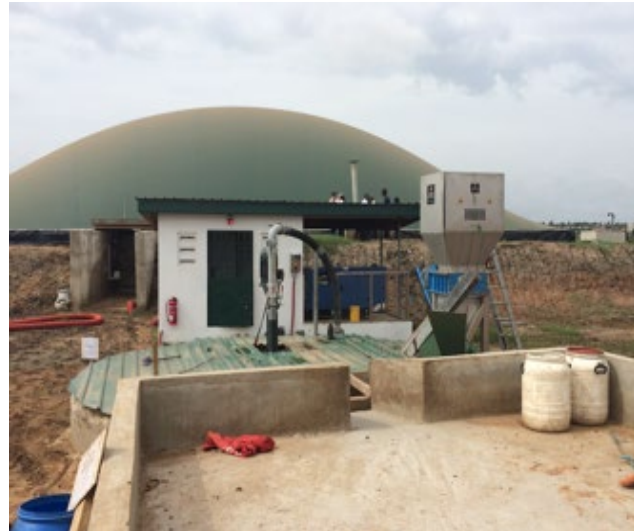
Mixing pit (fecal and organic waste) + macerator + digester
