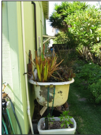
Figure 5. Recycled bathtub bio-filter for greywater system connected to drip, Beegril Gardens, Oakland, Calif.
