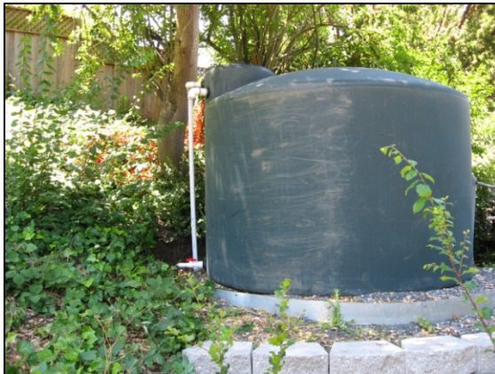
Figure 2. 2,500 gallon cistern storing water from roof in Figure 1
