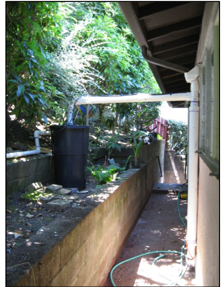
Figure 1. Rainwater catchment system installed by Planting Justice in Oakland, Calif.
