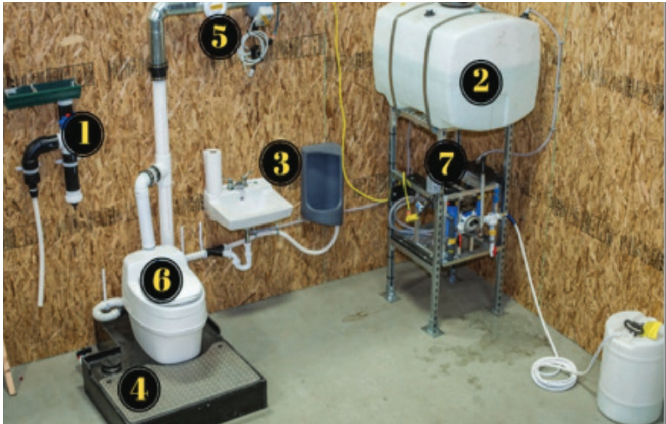
FIGURE 10. Portable Alternative Sanitation System
